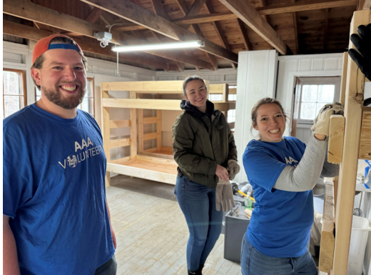
From left: Colin Benoit, Avery Owens, and Whitney Gerard building bunk beds at a summer camp.
